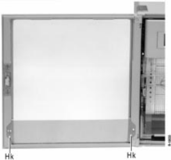
Figure 17 Replacing the label for measuring points at a door with metal frame
